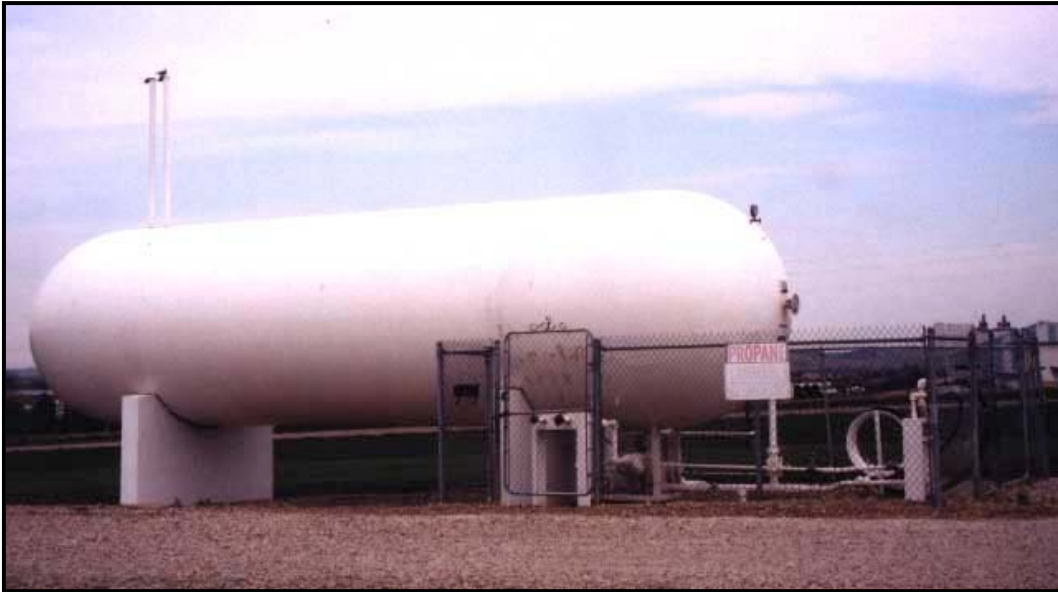
Figure F-9. 18,000-gallon liquid propane tank in industrial area.
