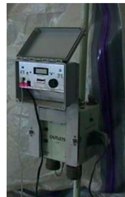
Pressure gauge with differential pressure alarms
